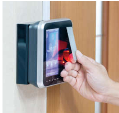
Access Control System
