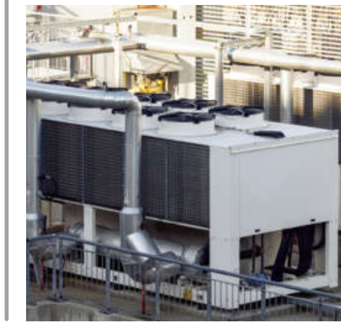
Chilled Water System
