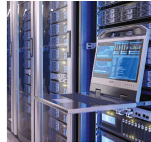
Server Room / Server Rack
